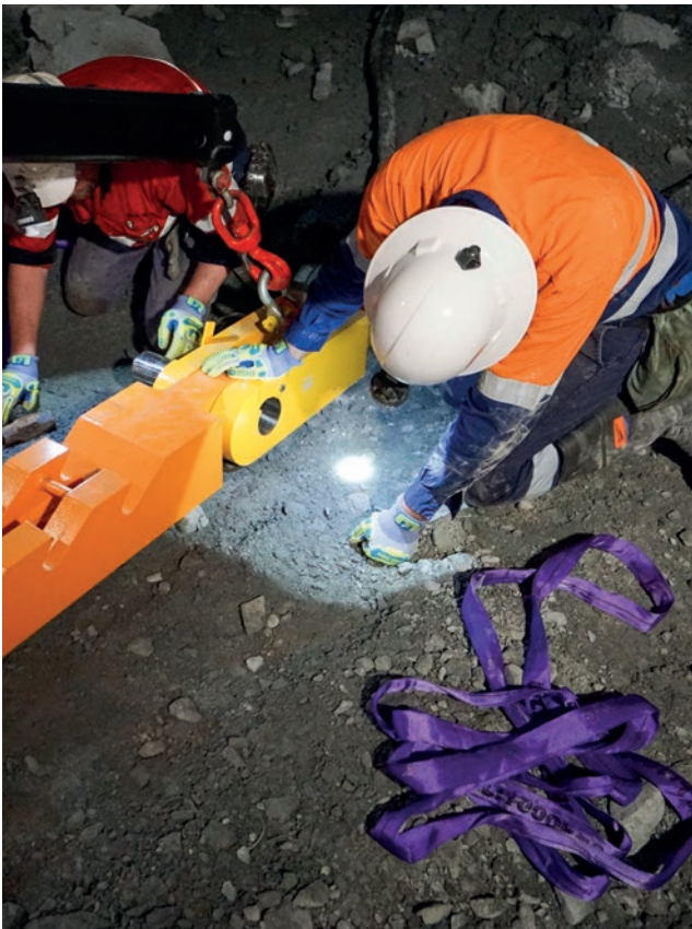
13. The connecting link is secured to the pulling rack using the load pin.
