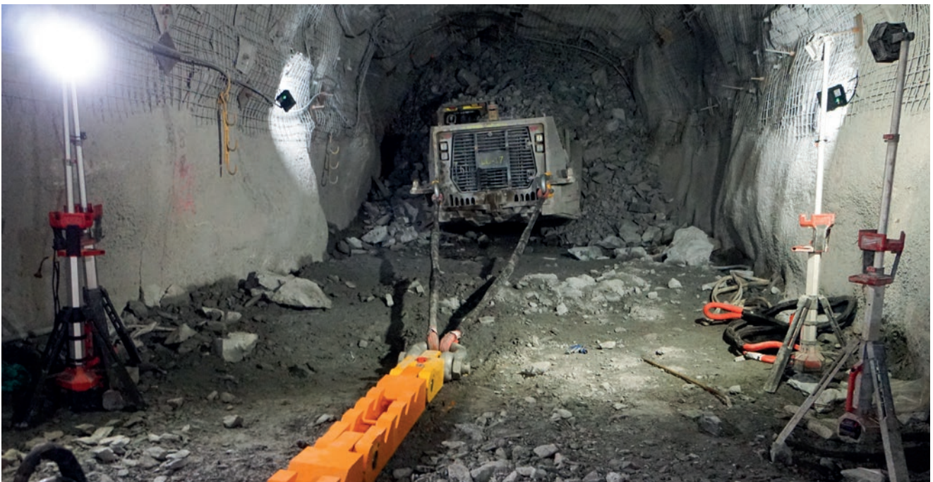
16. Tension is applied to the tow slings and the extraction process commences.
