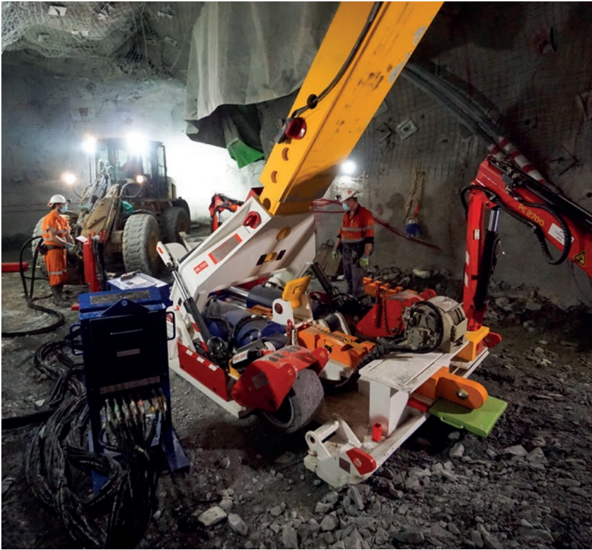
7. The control station and hydraulic hoses are moved into position and connected. In this case the auxiliary implement controls on an IT loader are used to operate the MED.
