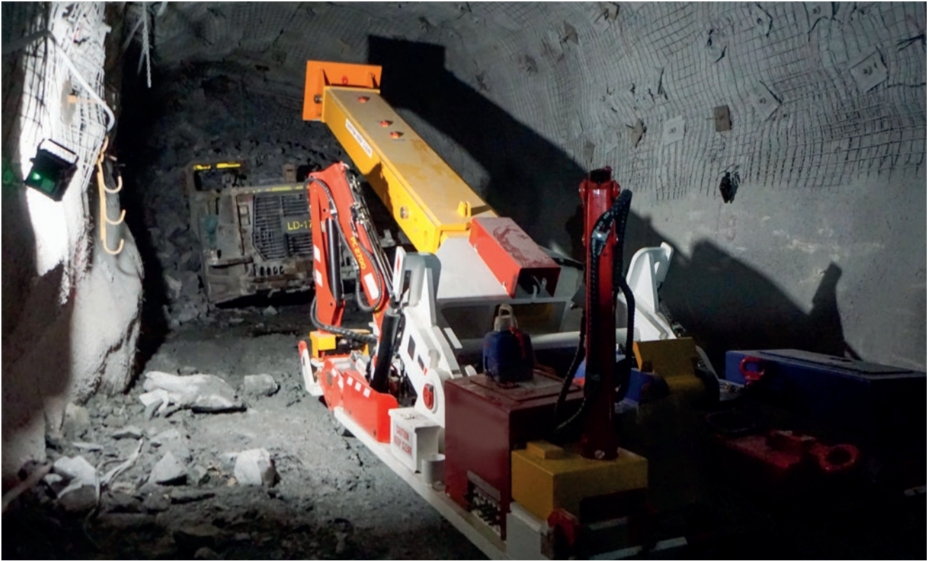
1. MED360 is being moved into place following the preparation of a solid and level base before the extraction commences.
