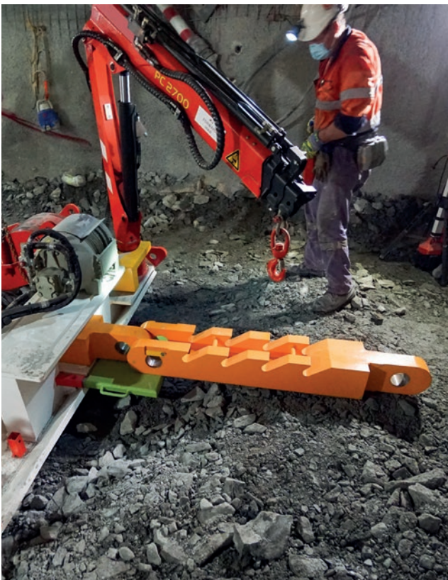
9. Racks are being located and pinned together using the front Hiab. (Hiab cranes are only available on the MED360).
